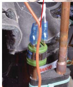
High Pressure Switch
