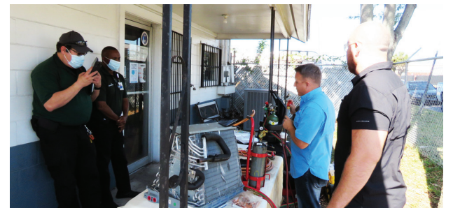
Ray Diaz and Fredrick Cintron of Advent Health with Chris Craft and Andres Ponce of Target Sales repairing an aluminum coil
